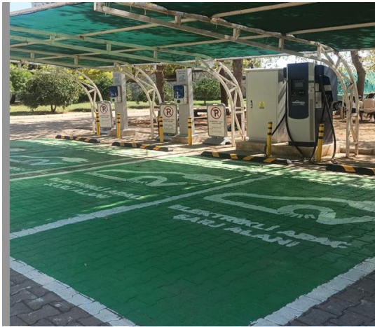
Example of Charging points for EV for cars (Akdeniz University, Türkiye)
