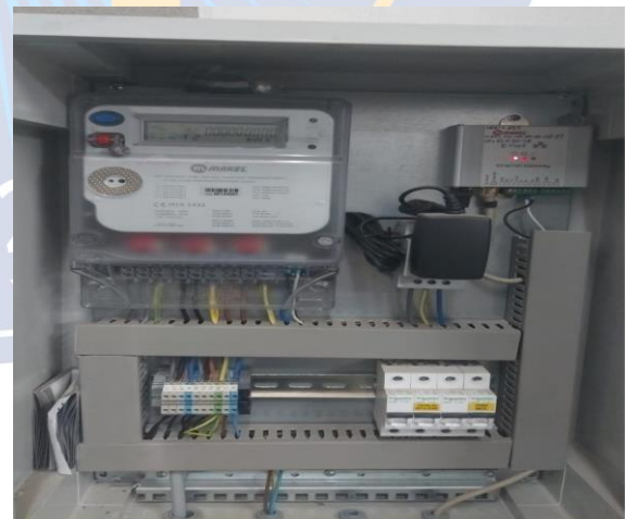
Example of Smart Meter Reading System
