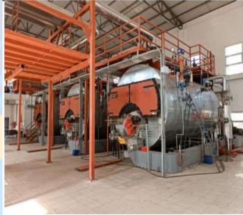
Boilers in Heat Power Station
