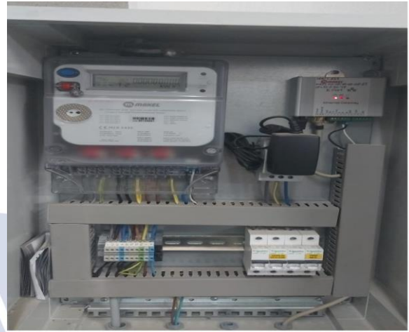
Example of Smart Meter Reading System (Makel Automatic Meter Reading System) Electrical Measurement Panel Used at Akdeniz University
